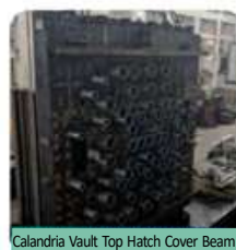
Calandria Vault Top Hatch Cover Beam
